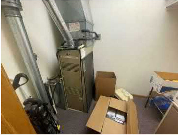
Photo #7 View of a gas furnace located in the front office.
