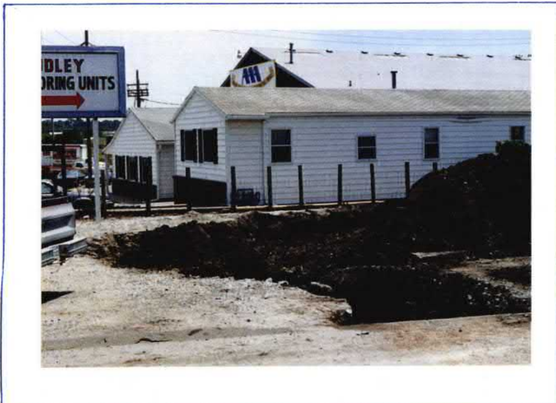
PHOTO 4. FACING EAST FROM WHERE FUEL ENTERED SOIL/CRUSHED ROCK AREA. PHOTO SHOWS EXCAVATION OF CONTAMINATED SOIL IN PROGRESS.
