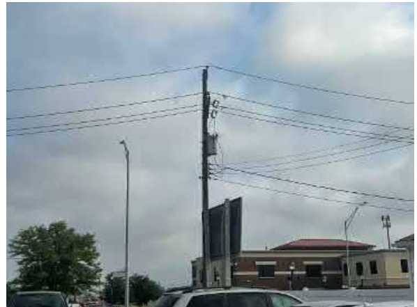
Photo #28 View of one of two pad-mounted transformers.
