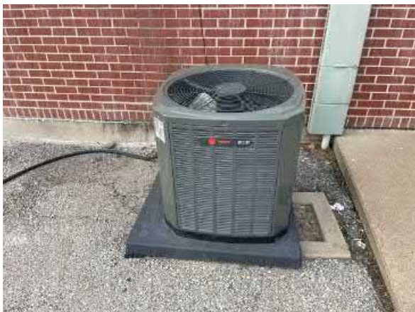
Photo #29 View of one of several air conditioning units for the front office.
