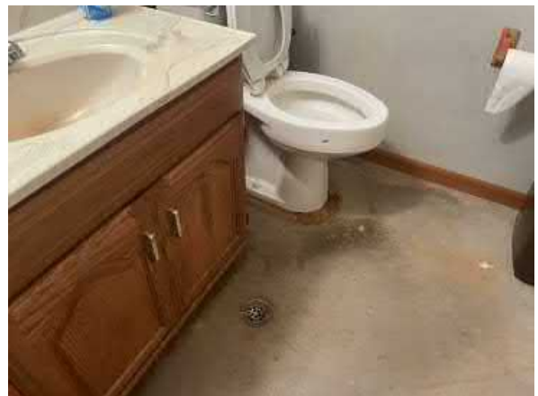
Photo #6 View of the floor drain located in the restrooms in the front office.
