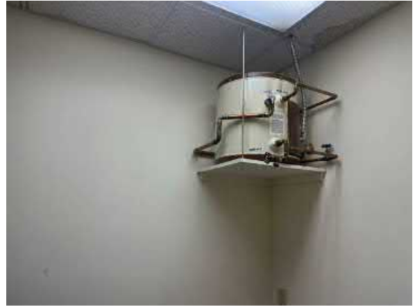
Photo #8 View of a suspended water heater located in the front office.
