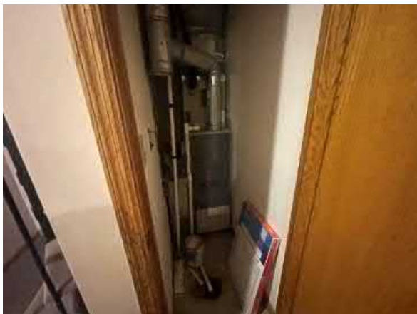
Photo #5 View of a furnace, paint can, and floor drain located in the front office of the site building.
