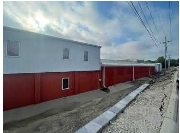
Photo #2 View of the site. View from the northwest toward the southeast.
