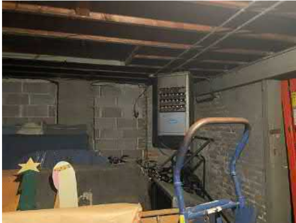
Photo #13 View of an out-of-use heating unit located in a storage warehouse.
