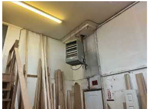
Photo #28 View of one of several natural gas heaters located throughout the southern site parcel buildings.
