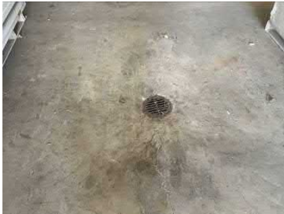
Photo #25 View of one of several floor drains located throughout the southern site parcel buildings.
