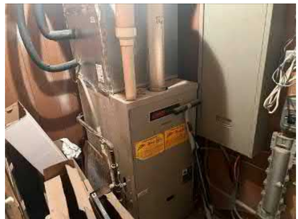
Photo #6 View of one of two furnaces that service the show room and sales offices.
