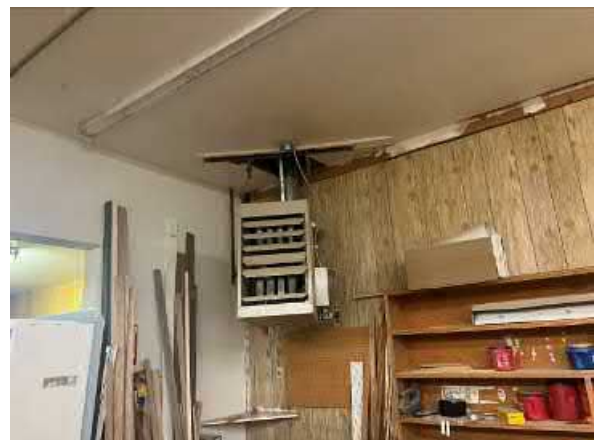
Photo #12 View of one of several natural gas heaters located throughout the warehouse space.
