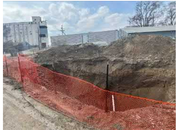
Photo #16 View of City of Ralston utility work excavation located on the southern end of the northern site parcel.
