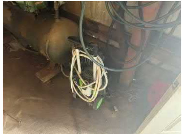
Photo #26 View of an air compressor and de minimis staining located in one of the southern site parcel buildings.
